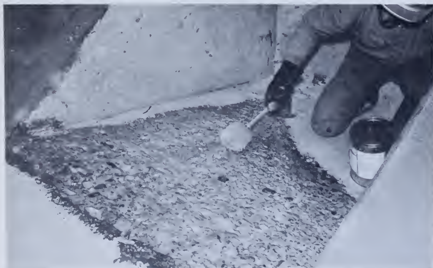
Figure 182.—Epoxy bond-coat being applied to sandblasted area adjacent to the dentates in Yellowtail Afterbay Dam sluiceway. Following this, epoxy mortar is placed over fluid or tacky epoxy to form epoxy-bonded epoxy mortar. P459-D-68900.
